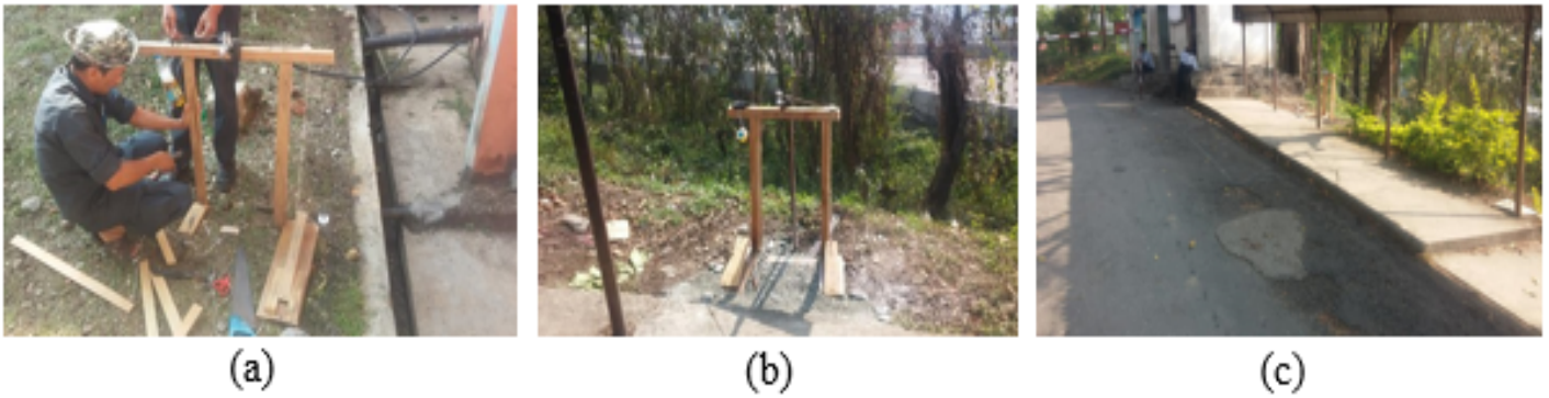
Figure 3 (a) Foot operated faucet hand was station under construction, (b) installed foot operated hand was station, and (c) location of installed hand wash station at the gate of the college.
